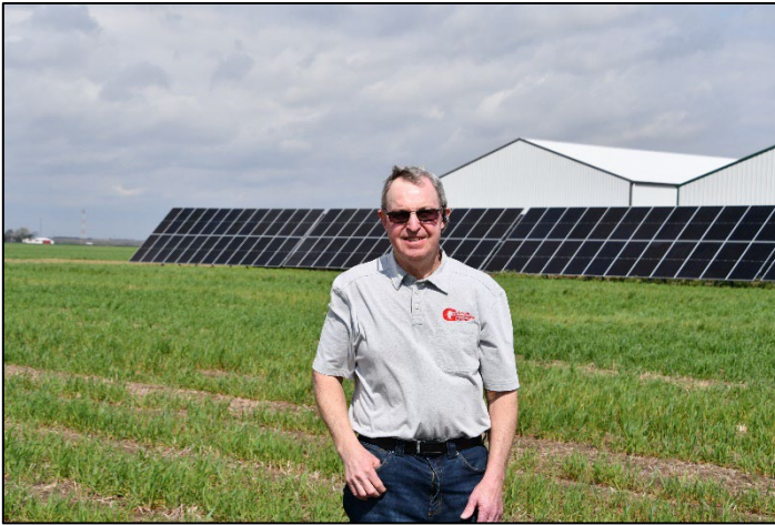
Doug Goyings stands near the ground-mounted solar array he installed on his northwest Ohio grain farm with help from a USDA Rural Energy for America Program grant. USDA Photo.
