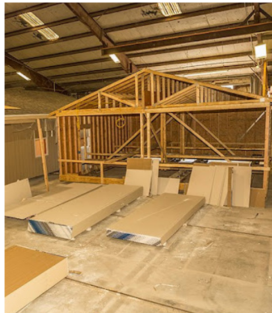
Example of modular home under construction, Advanced Systems Homes located in Chanute, KS. | Image courtesy of Advanced Systems Homes
