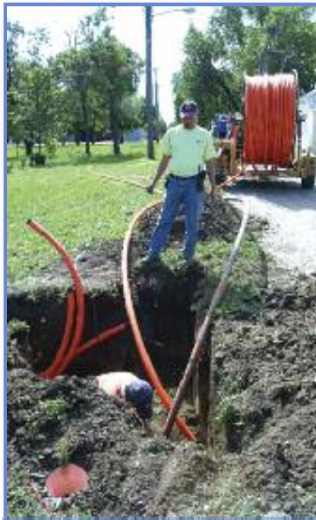
New broadband lines are being installed by the BEK Communications Cooperative in Burleigh County, N.D. The $6 million project is being supported with loan and grant money from USDA. Photo courtesy BEK Communications
